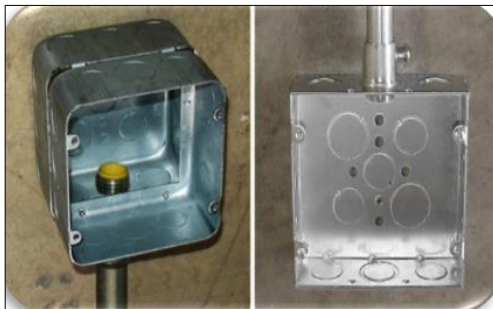
Fig 11: Wall recess mounted Outlet
