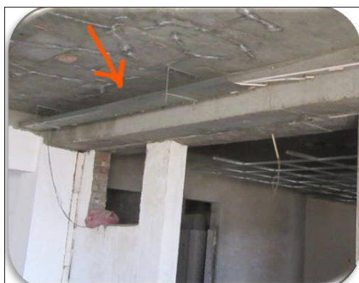
Fig 8: Elevated Pathway (cable tray)
